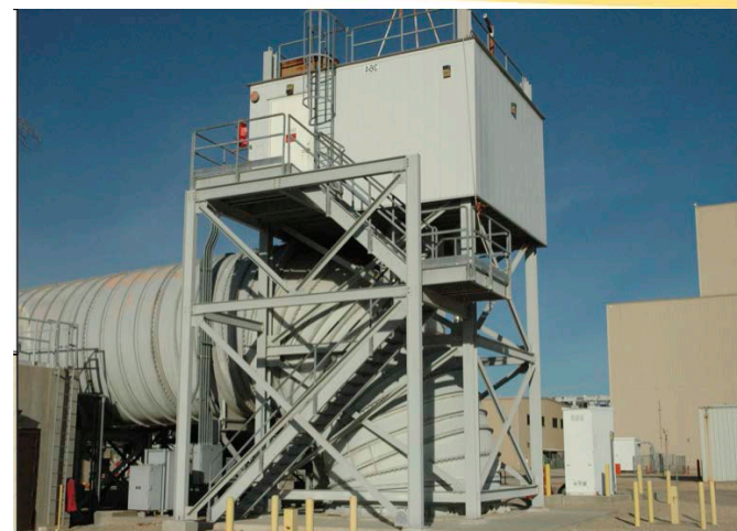
Station A, Fixed Air Sampler
